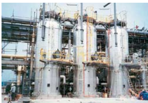
Feed Gas Dryer
